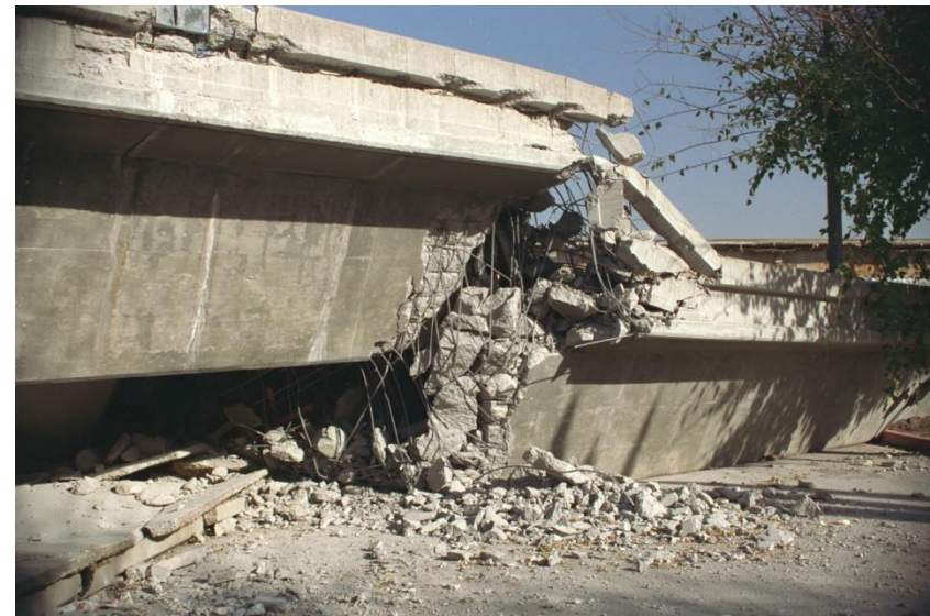
Failure of primary- and secondary structure
