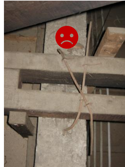
Roof tension anchor?
