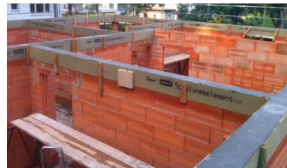
Masonry wall head not secured, Ring anchor is missing
